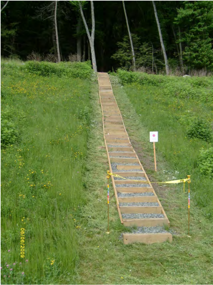
Steps constructed by ITTF down embankment to Rte 7 (l) view from Pine Mountain (r)
